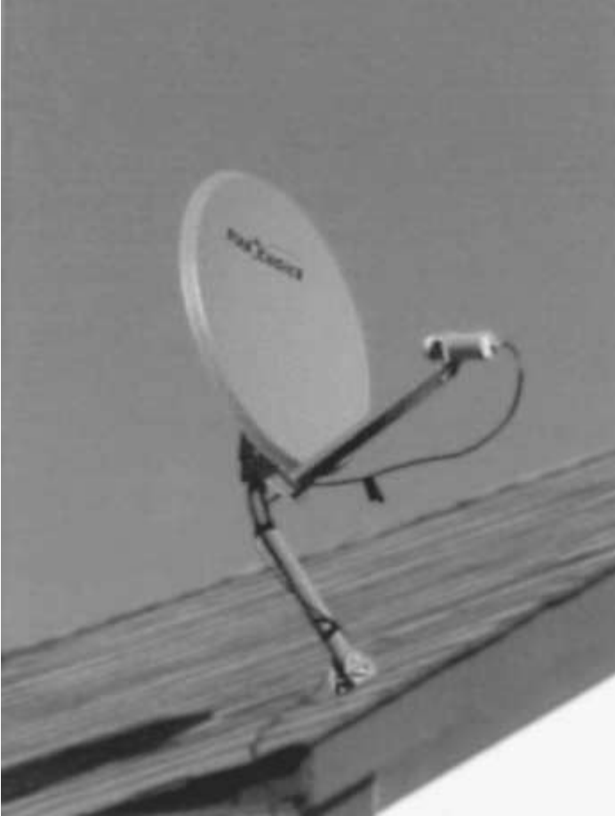
Figure 16.6 A typical DBS antenna installation.
